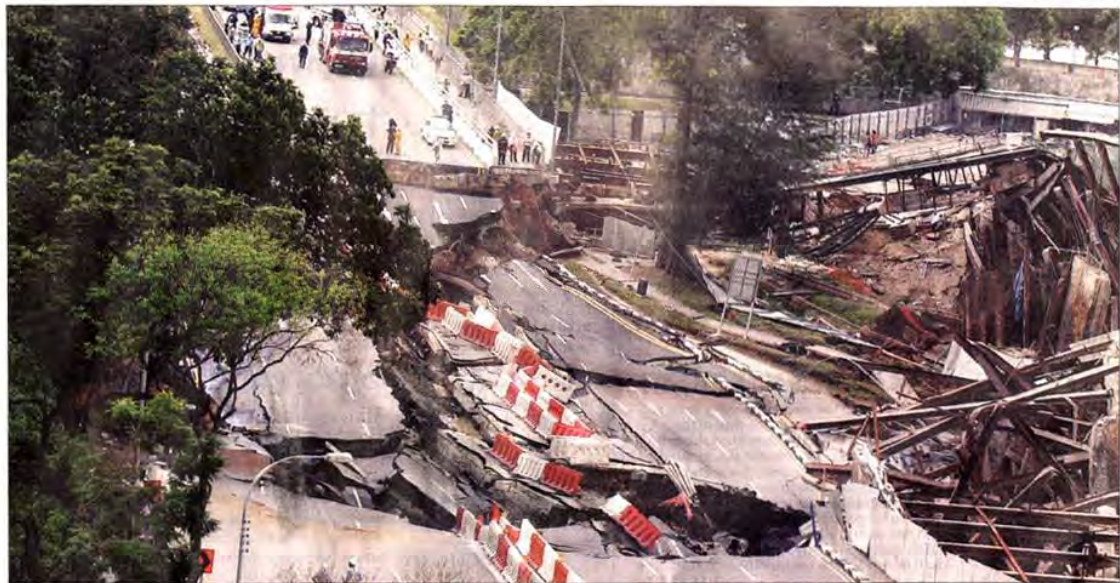
A 30m-deep ravine opened up within minutes of the first collapse, which has initially been blamed on a temporary supporting wall.
